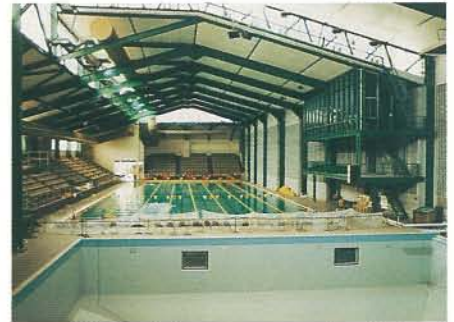
X. A vapour seal is provided as well as structural steel protected by ENVELON in a warm chlorinated environment
